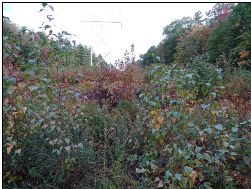
Figure 13. Shrubland habitat is maintained along the utility right-of-way at the Horse Hill Nature Preserve. This habitat is declining in the state and provides critical habitat for a variety of wildlife and plants.
